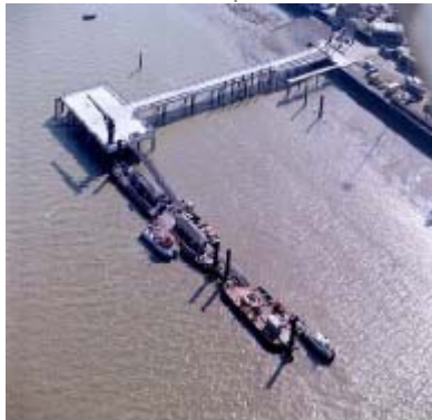
Denton Wharf Project, London Haswell have been appointed as a Civil/structural and Electrical Consultants to the Port of London Authority for the demolition and re-construction of Denton Wharf
