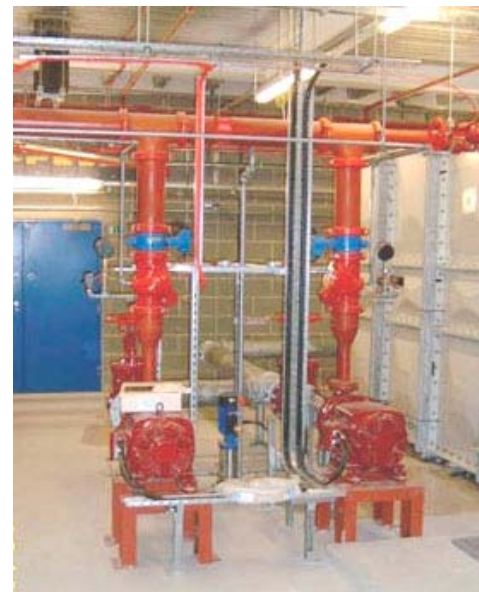
Completed Plant Room (April 2005)
