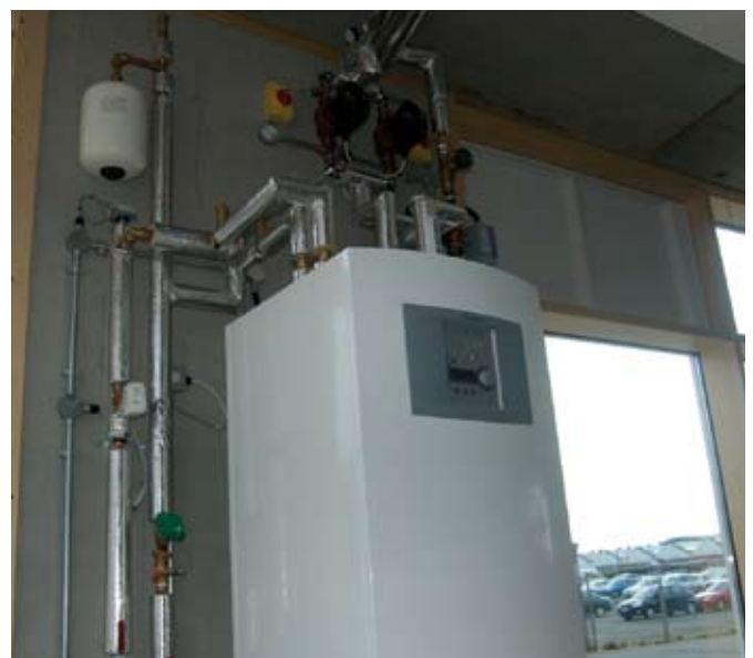
Worcester Ground source heatpump
