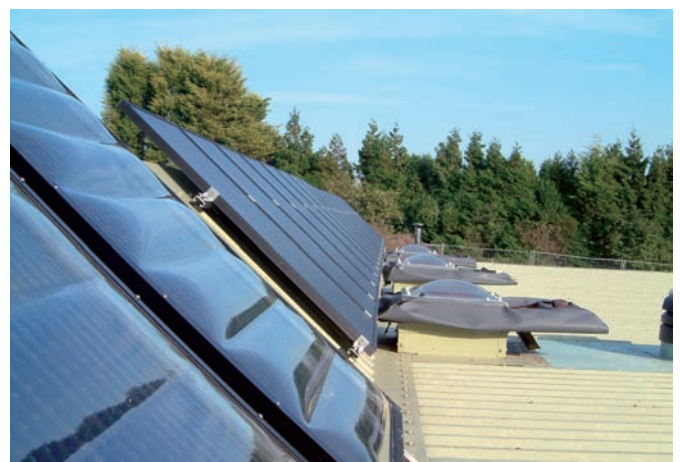
Solar panels at Earthship Brighton
